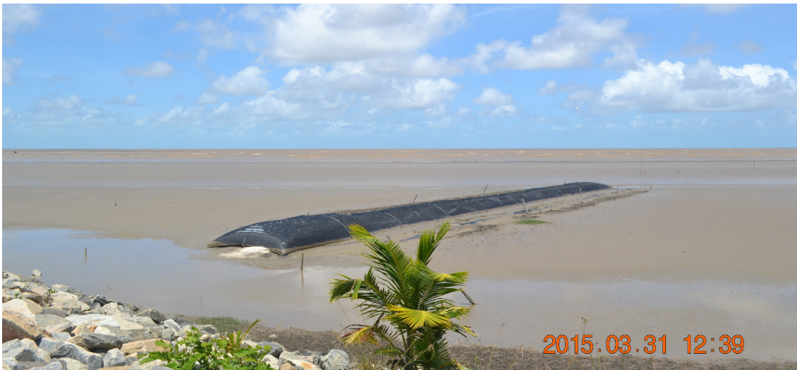
Figure 20.32 Site conditions following completion of a geotextile tube groyne at Devonshire Castle (Guyana), Region 22014. (Credit: L. Jack, NAREI)
