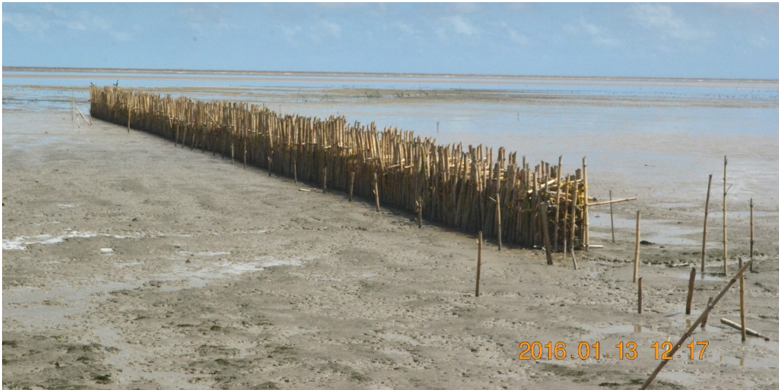
Figure 20.31 Brushwood dam constructed at Walton Hall (Essequibo Coast, Guyana), Region #2 in 2015. (Credit: L. Jack, NAREI)
