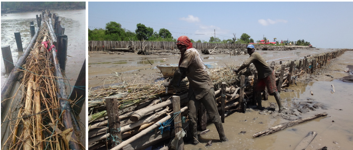
Figure 20.36 Construction of the sediment trapping unit at Weg naar Zee, Suriname, in September 2015. Left: top view of the dam structure (see text for details). (Credit: C. Fung-A-Loi and S. Naipal, AdeKUS)
