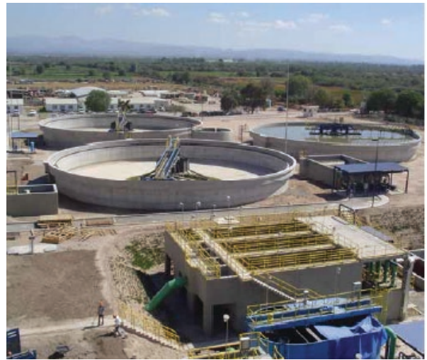
PHOTO 1. Tenorio Wastewater Treatment Plant
