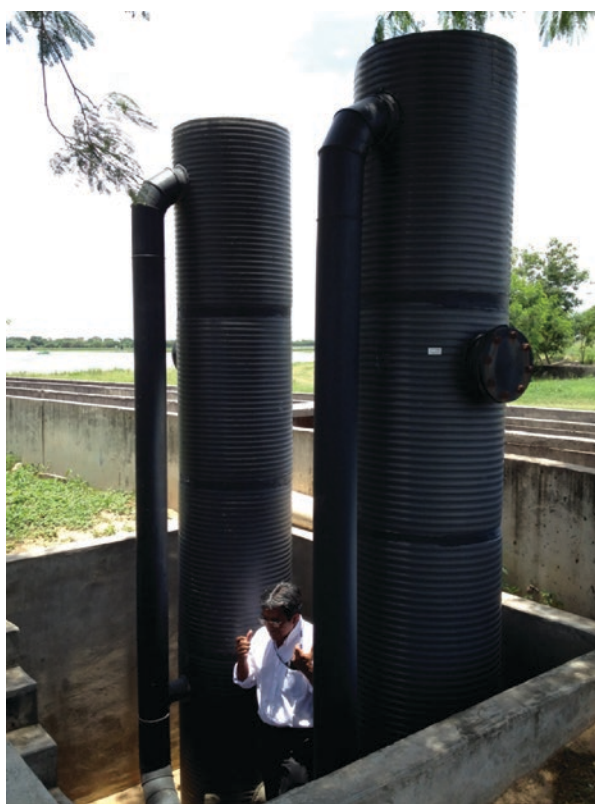
PHOTO 2. Water Traps at Biogas Line at SAGUAPAC WWTP
