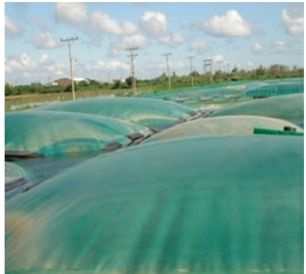
PHOTO 1. SAGUAPAC WWTP's Anaerobic Lagoons Covered to Collect Biogas and Reduce Odors Generated During Anaerobic Metabolization
