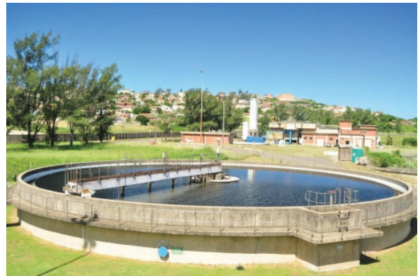
PHOTO 1. Durban Water Recycling Plant
